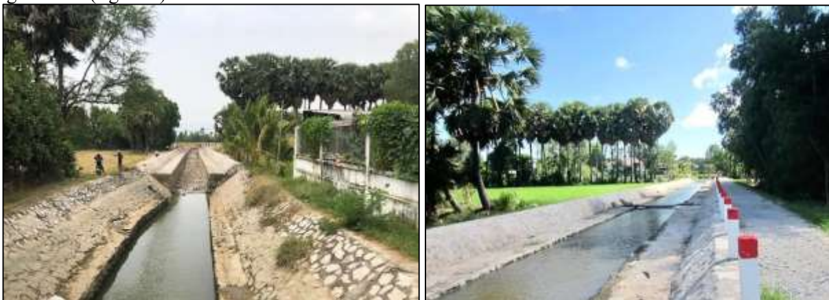
Figure 8. Canal under construction (left picture) and completed canal delivering water to the rice fields (right picture) in Van Giao Commune, Tinh Bien district.
